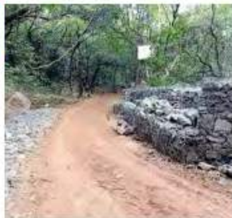
Work order for Dasturi to Matheran pathway and parking work was issued in September 2019
